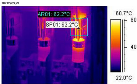
Figure 13.3 An infrared image of a fusebox where the maximum temperature is displayed
